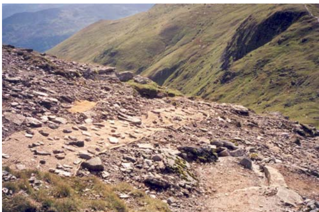
Photo 2 Coir and jute netting laid adjacent to Ben Lawers main path. Photo by Helen Cole
