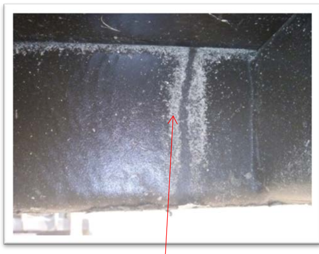
Figure 3. Evidence of ant galleries
