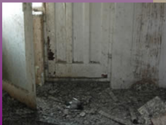
Damage done by Pigeons to a derelict building Photo: rpcwildlife.co.uk
