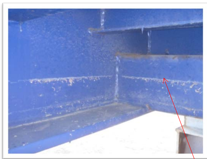
Figure 2. Evidence of organic material from water high tide mark
